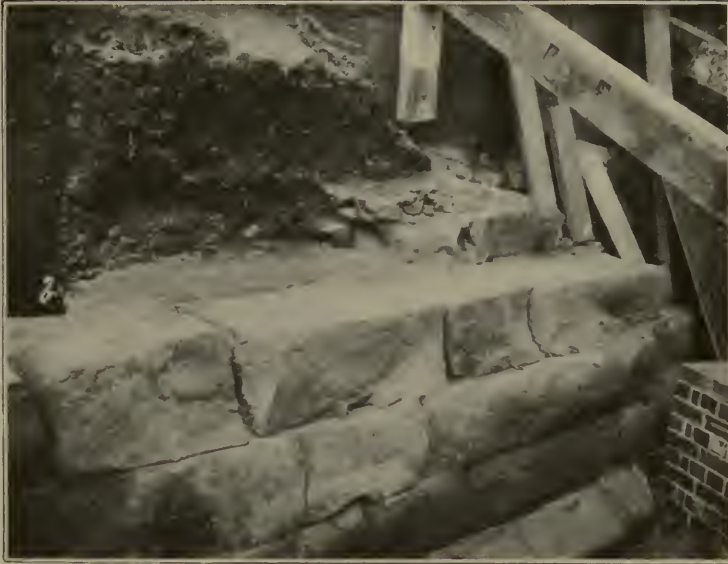
FIG. 1.—ROMAN WALL (PORTION AT NORTH END) SHOWING AT b THE COURSING OF THE RUBBLE WORK.
